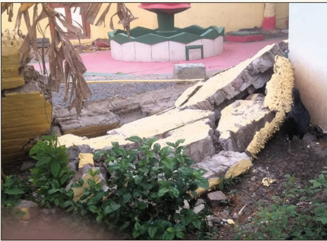
Collapsed wall at the Church of the Lutheran Confession, India
