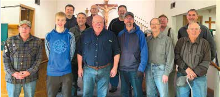
Above: Members of Messiah, Eau Claire, help St. Paul's members move pews to clear the way for ceiling repairs.
