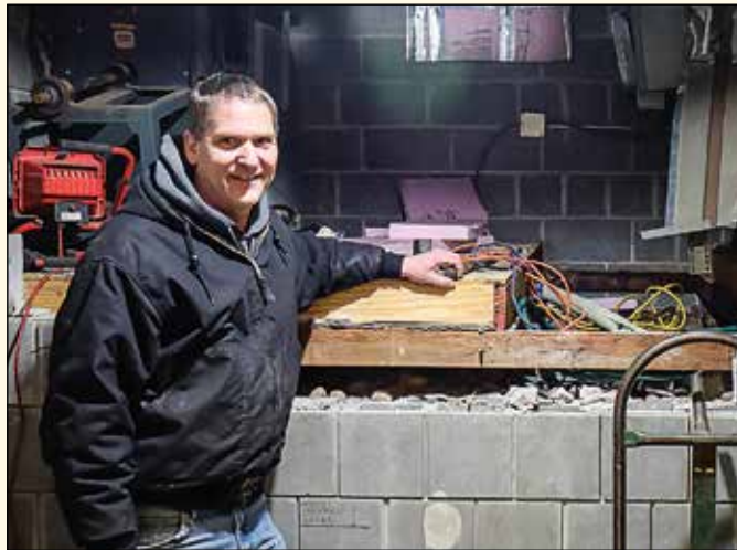
Top: North Hall, the boys' dormitory. Above: facilities manager Paul Heinze showing where the new boiler will be installed.
