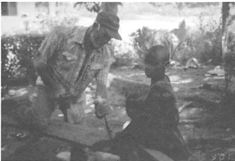
Up to 18 volunteers each day helped Larry (shown here) and Martin Hansen (below) in their remodeling project in Nigeria (see picture, p.13).
